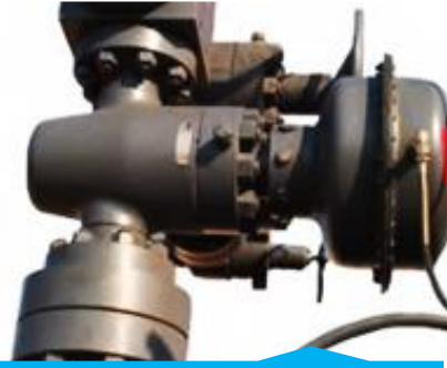
O&G valves and wellheads
